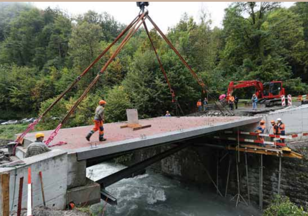
This 11.4-meter long bridge in Bex, Switzerland, featuring a balsa wood core, was installed as a single piece in less than three hours.
